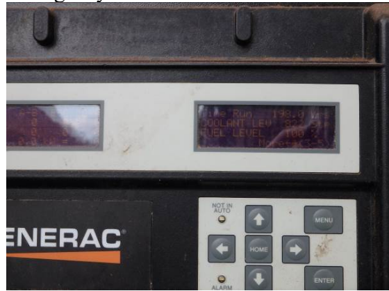
16) Emergency Generator Panel
