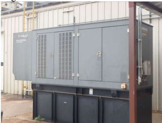
15) 402 HP Emergency Generator Engine
