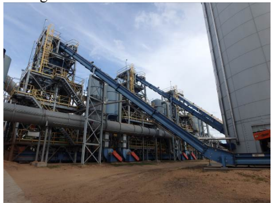
12) 3 Hammermill Pneumatic Systems w/ Baghouse
