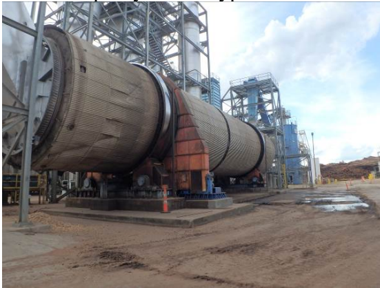
14) Wood Chip Dryer and Bypass Stack
