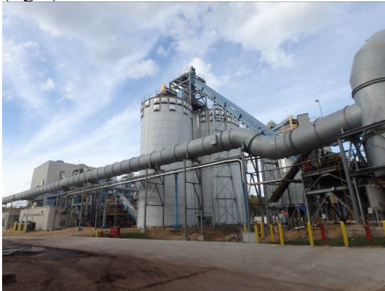
13) Dry Fiber Silo 1 (left) and Silo 2 (right) w/ Bin Vent
