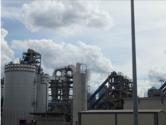
1) Storage Silo w/ Bin Vent
