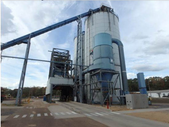
2) Pellet Storage Silo and Pellet Truck Loadout System
