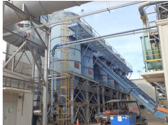
17) Pellet Mill/Cooler Pneumatic Systems
