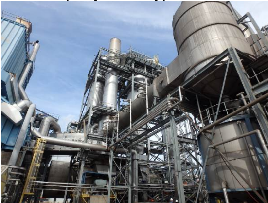
8) Wood Chip Dryer and Bypass Stack
