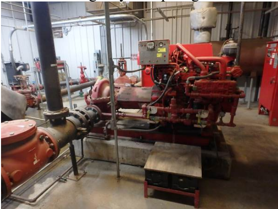
21) 250 HP Emergency Pump Engine
