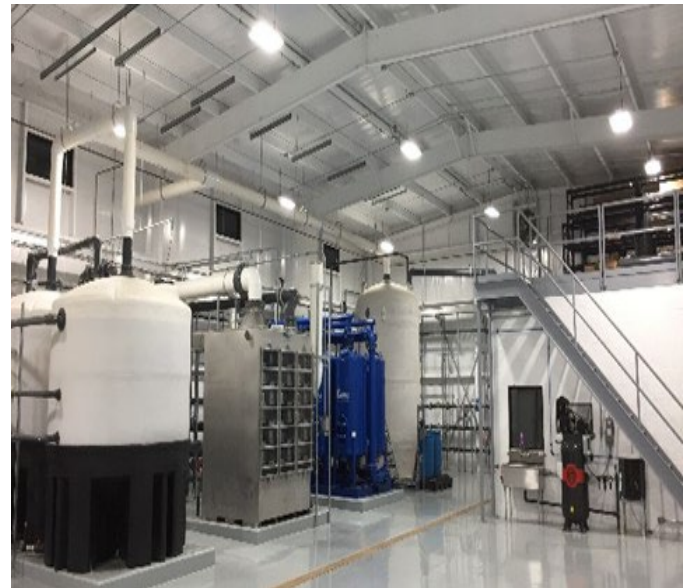
A view inside of the Facility P&T groundwater treatment building.
