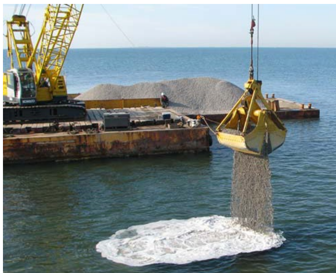
Existing artificial reef areas (each approximately three acres in size) enhanced with clean, crushed limestone.
