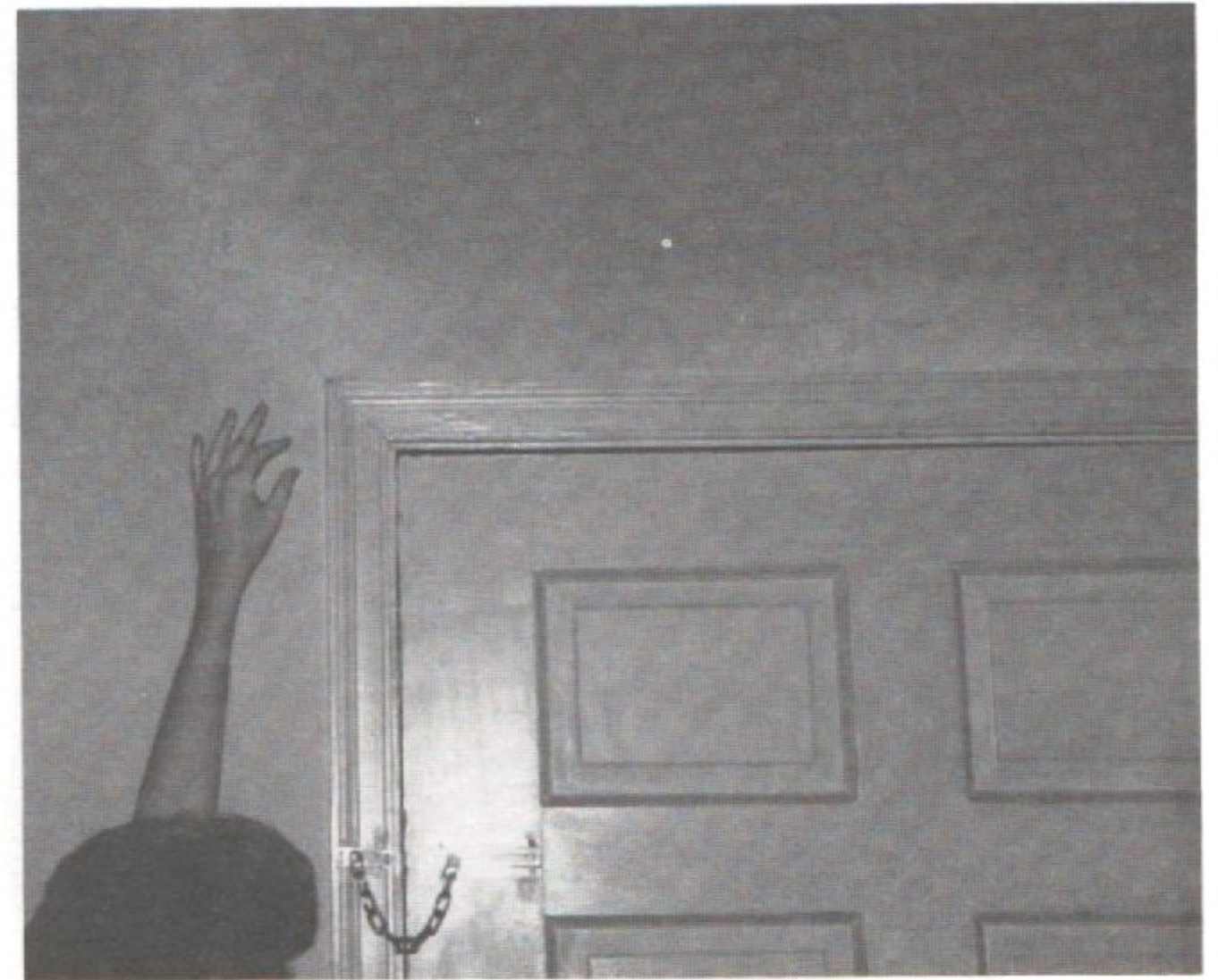
Figure 18. Common inside house damage.
