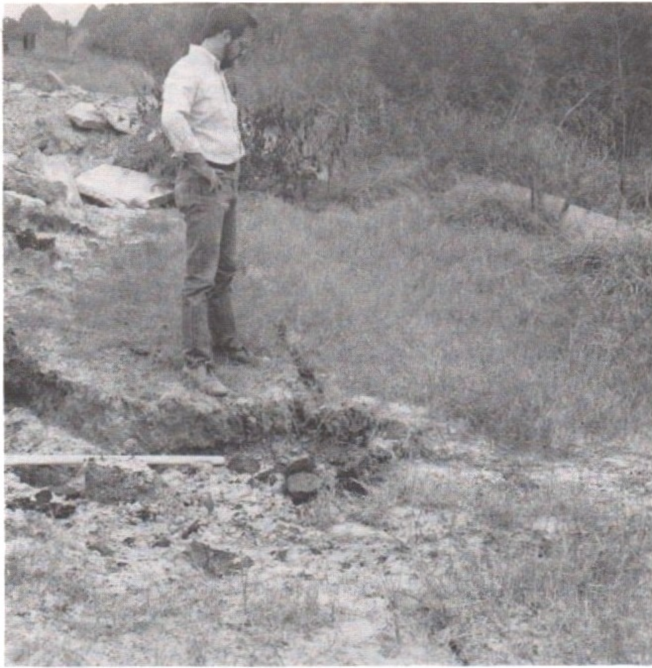
Figure 26. Example of slide along a drainage ditch.
