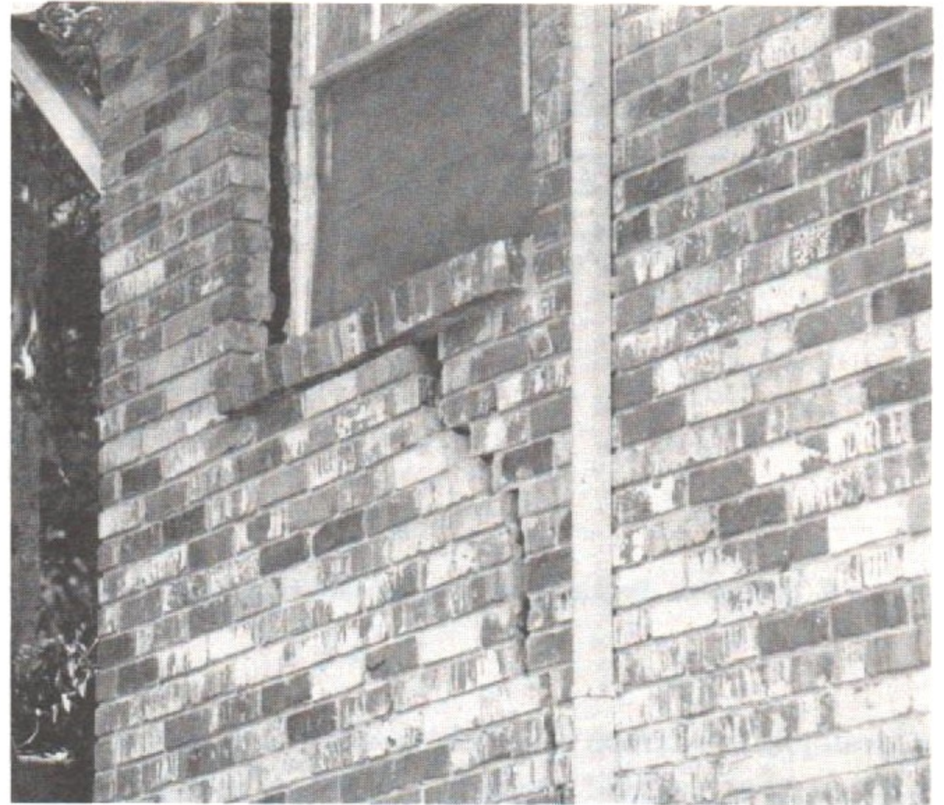
Figure 11. Apartment building, second level, with horizontal displacement due to differential vertical movement of the soil.
