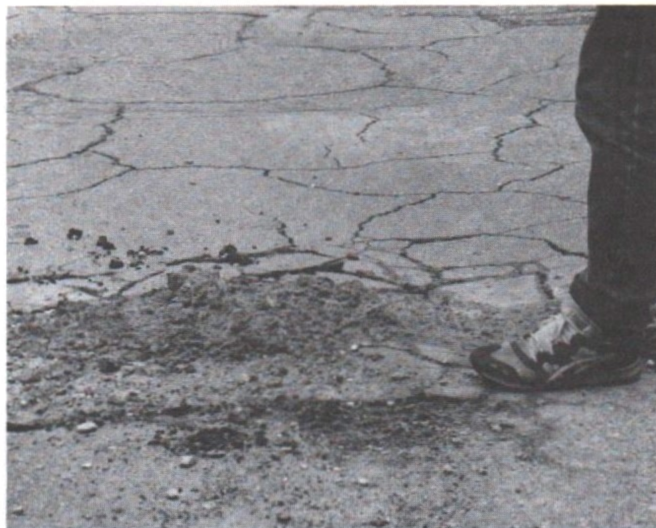
Figure 22. Example of damage done to roadway caused by allowing water to seep underneath.
