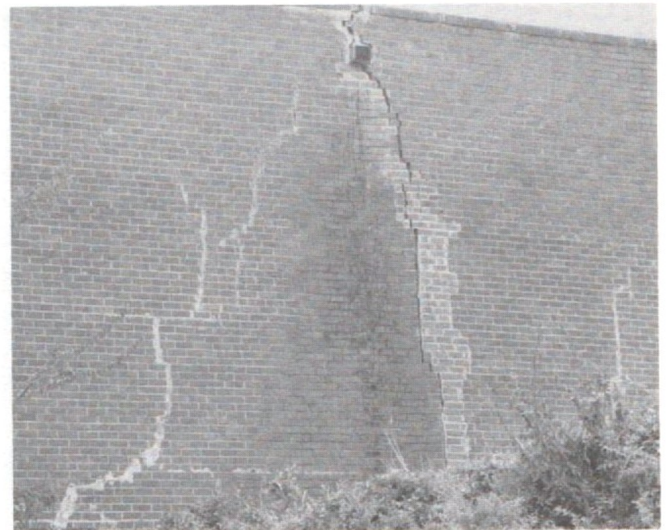
Figure 19. Building with wall cracked from foundation to roof.
