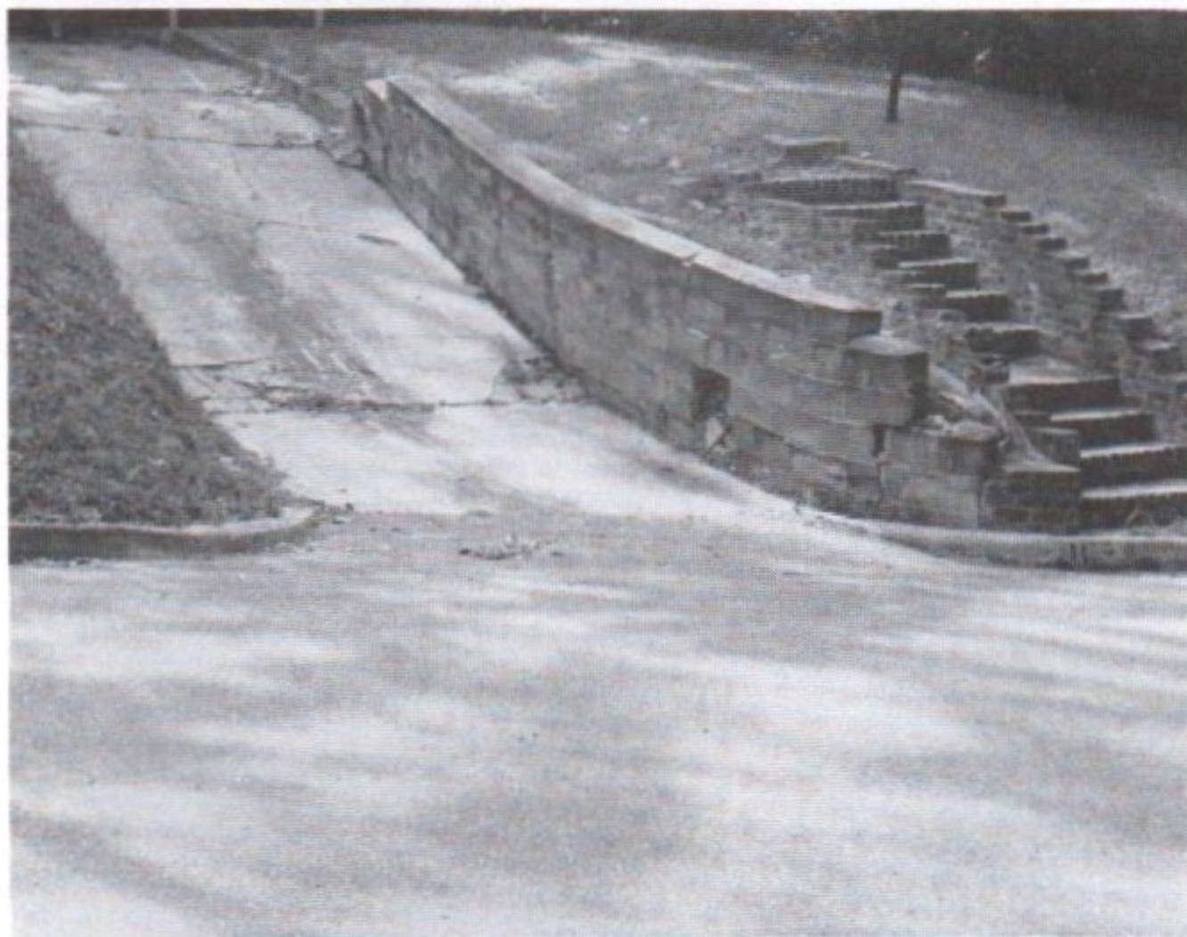
Figure 21. Horizontal and vertical movement damaging retaining wall and driveway.
