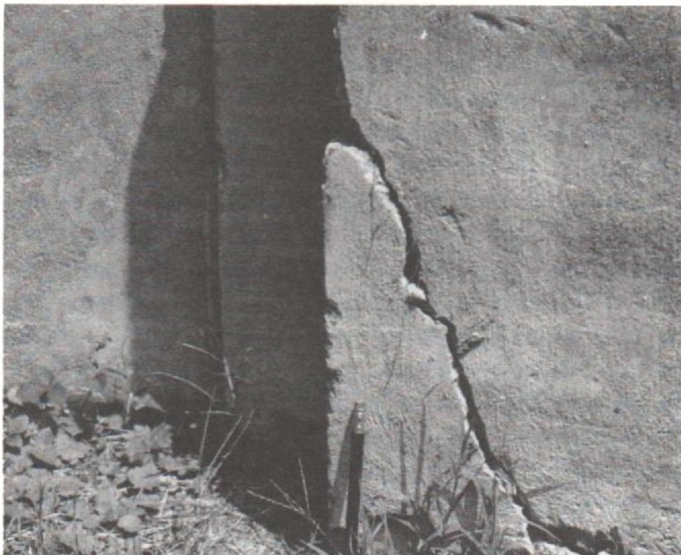
Figure 9. Building pier with vertical and horizontal displacement.
