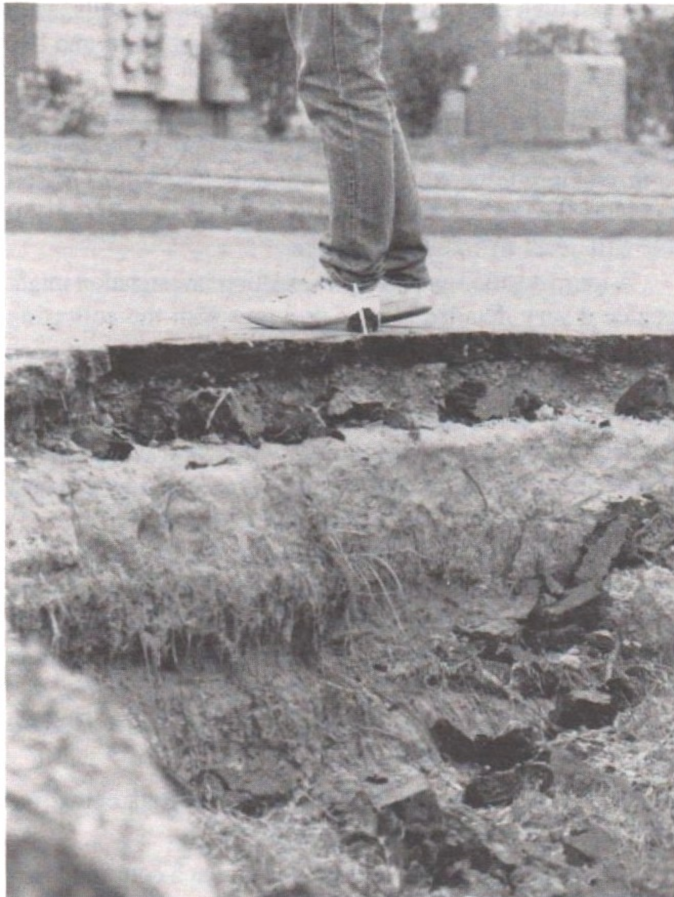
Figure 27. Example of slide and the damage done to roadway.
