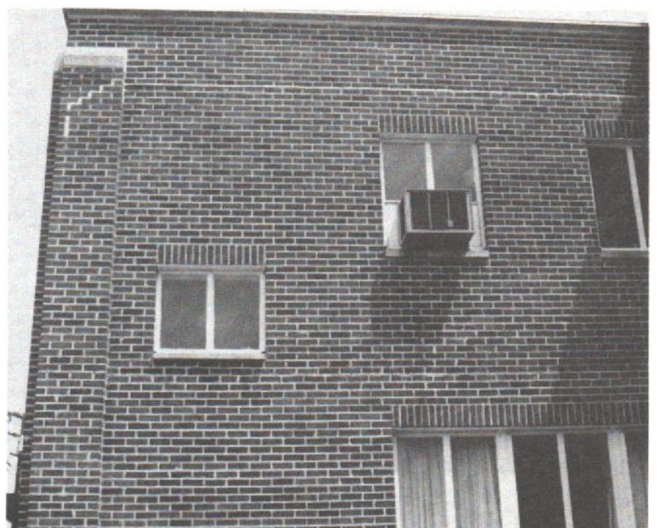
Figure 13. Building pier, third level, with horizontal and vertical displacement.
