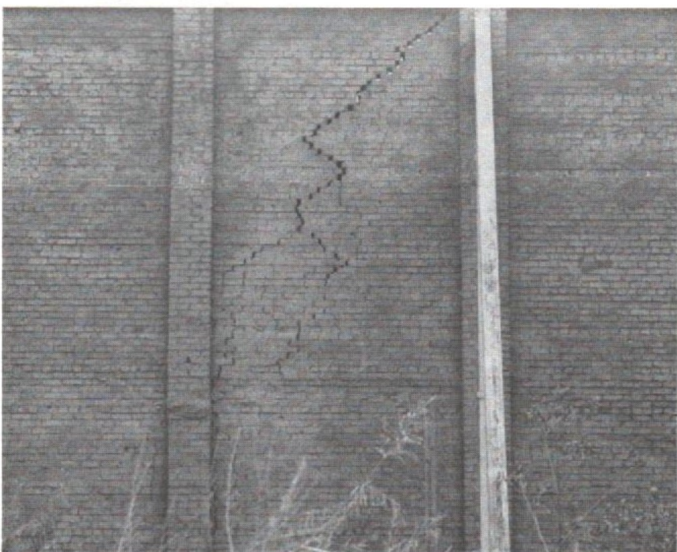
Figure 10. Brick wall with horizontal displacement due to differential vertical movement of the soil.
