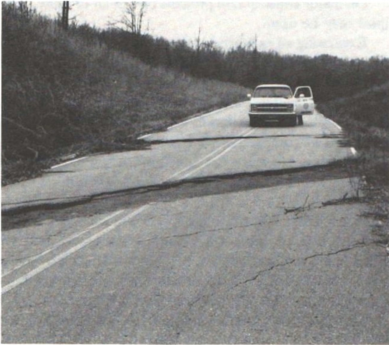
Figure 23. Highway damage caused by massive slide.
