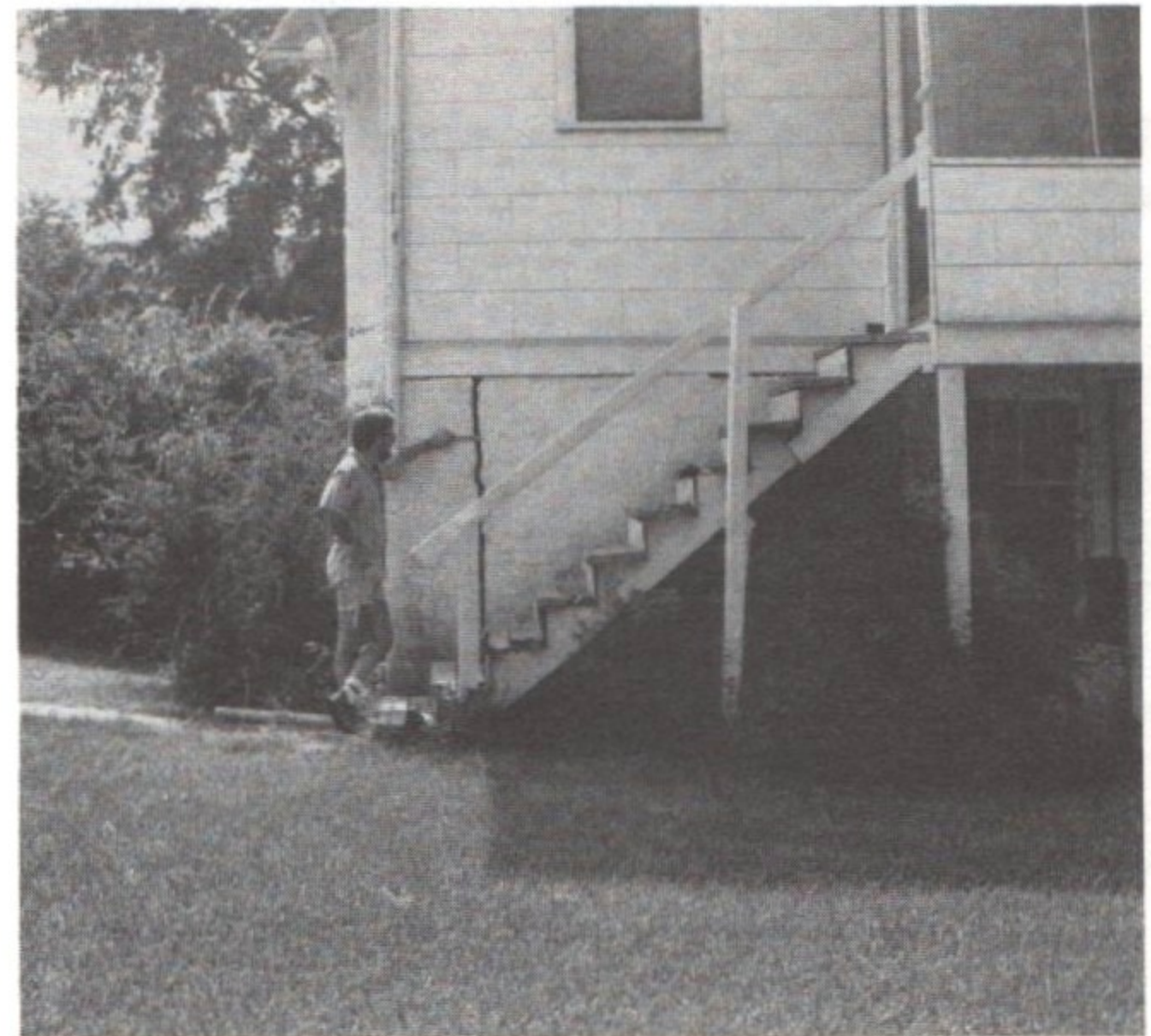
Figure 7. House pier with horizontal displacement indicated by pointer.
