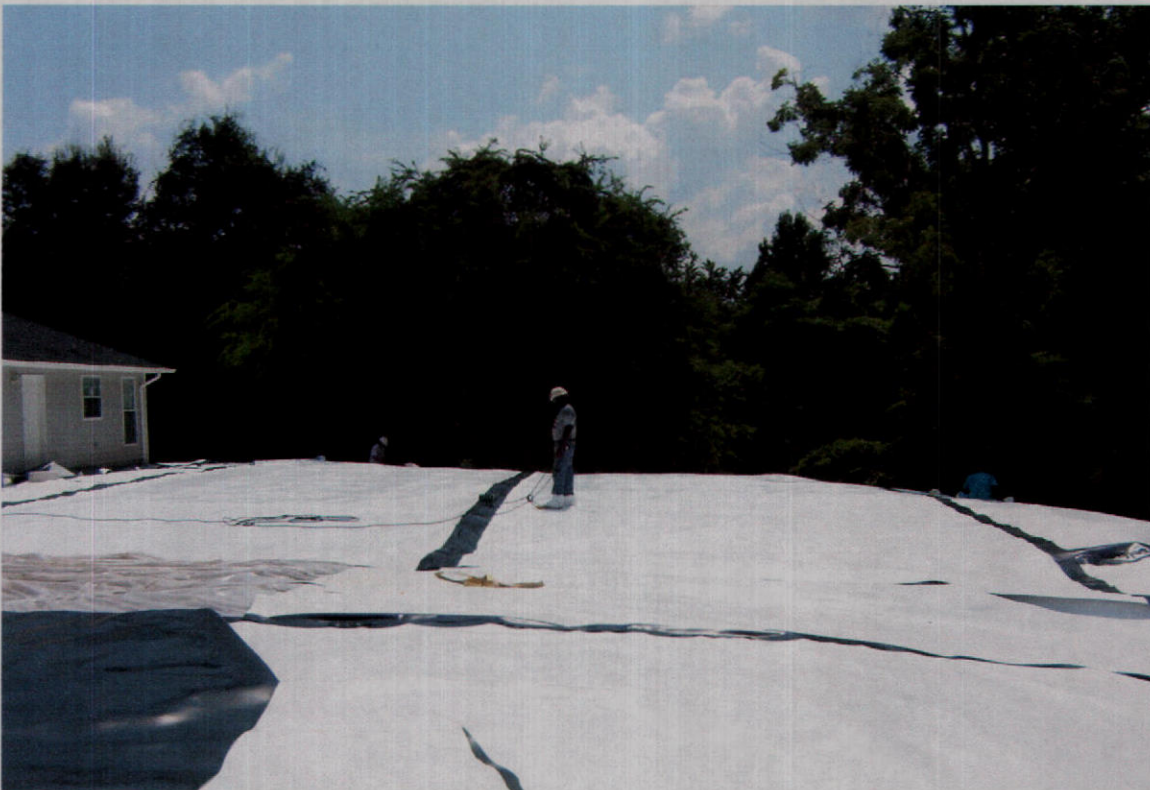
PHOTO 2 – Workers completing the installation of the LDPE protective liner at 114 Brent Street. Photo was taken looking north to south.
