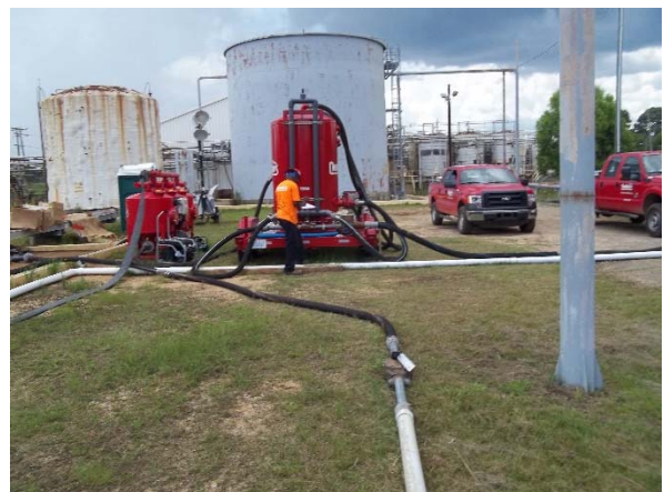
Carbon treatment of water
