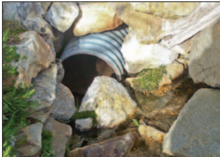
Figure 34—Rock failure around an outlet pipe.
