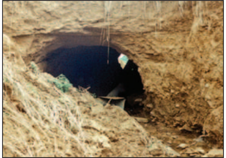
Figure 32—Piping of water alongside an outlet pipe.
