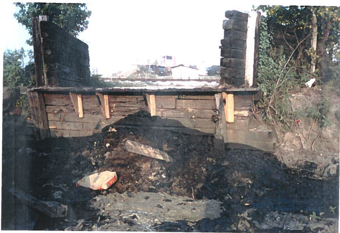
Photo № 21 Roll № 1 Frame №: 23 Date: 6/25/92 Subject: The unloading dock located near the drum recycling area. Location of HI-SS-02. Notice the stained soil and stressed vegetation.
