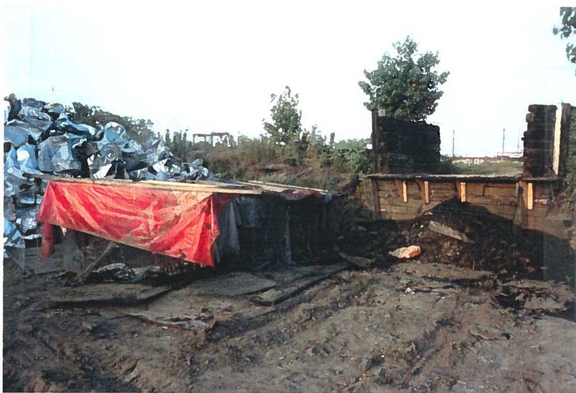
Photo № 22 Roll № 1 Frame №: 24 Date: 6/25/92 Subject: Dumpster on left (covered with a tarp) which has been filled off the unloading dock. Note: Dumpster was removed, area was "clean" during the second site visit in August 1992.
