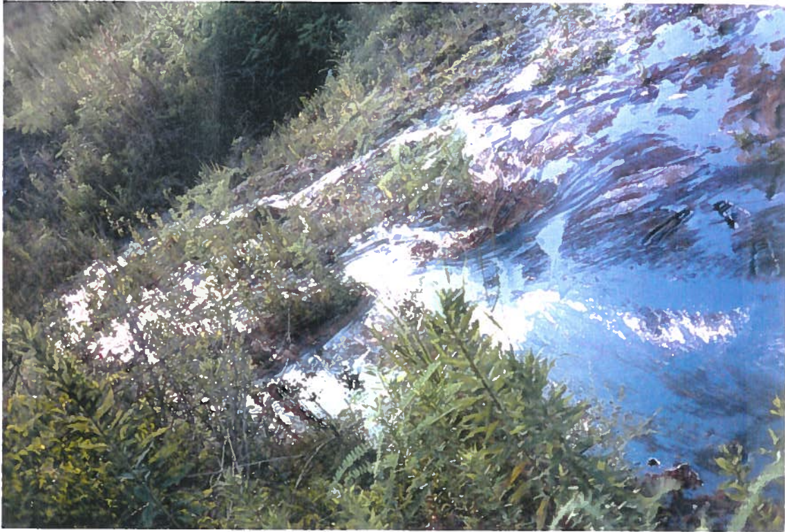
Photo № 16 Roll № 1 Frame №: 17 Date: 6/25/92 Subject: Sludge pit material that has flowed out of the diked areas, and has hardened. This sludge exhibits increased viscosity with ambient temperature.
