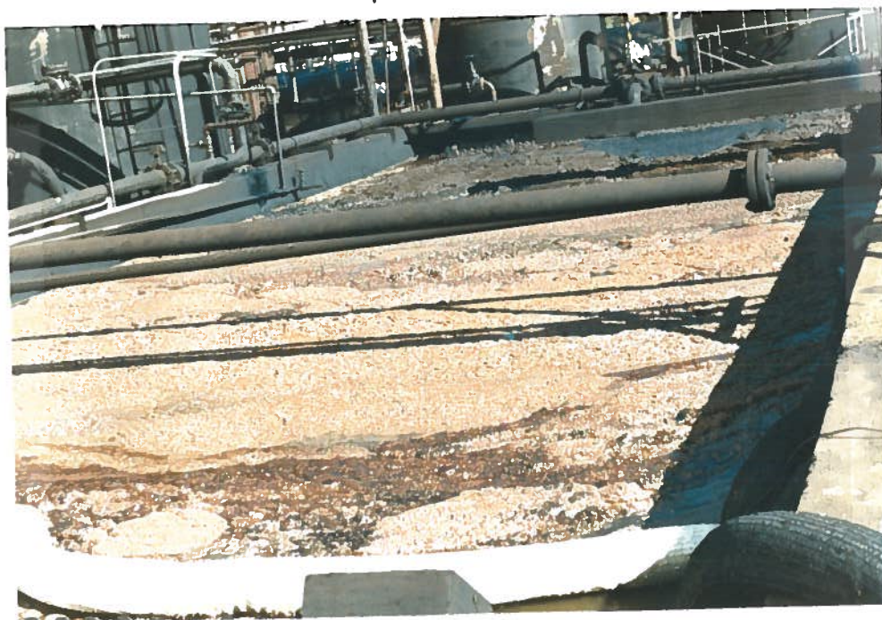
Koppers Co. Inc. Grenada (Die Plant) Facility API Separator ("Left-hand" tank, if you are facing east.) 12/19/85 Inspection by Jim Hardage
